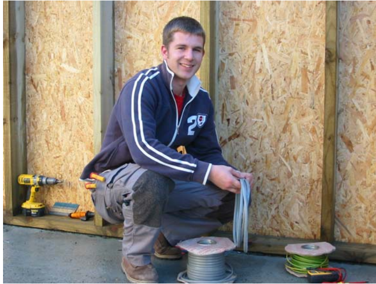
Photo:- Donald Macrury, D Macrury Electrical
